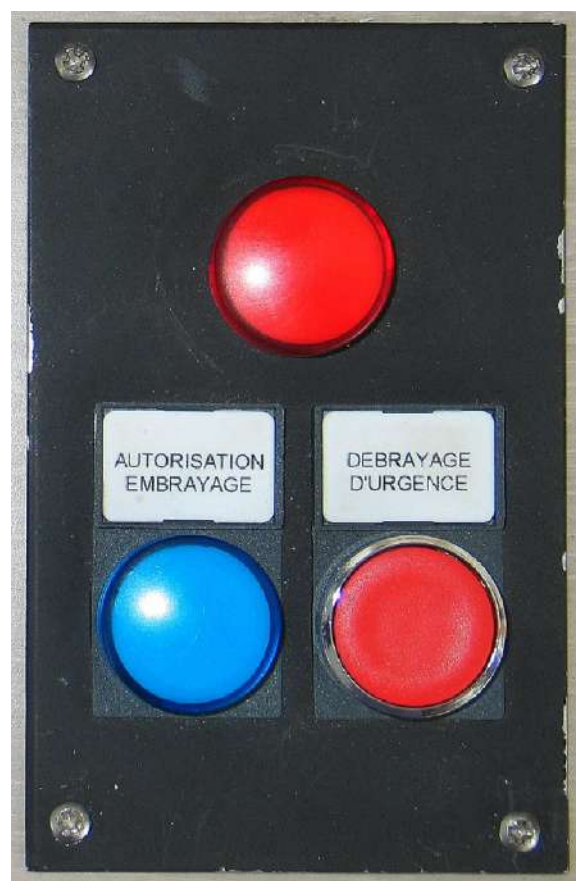
Figure5-40 Bridge - Gearbox Clutching Remote Control Panel
