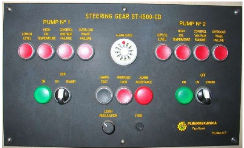
Fig5-2 Bridge - Steering Gear Remote Control Monitoring and Alarm Panel
