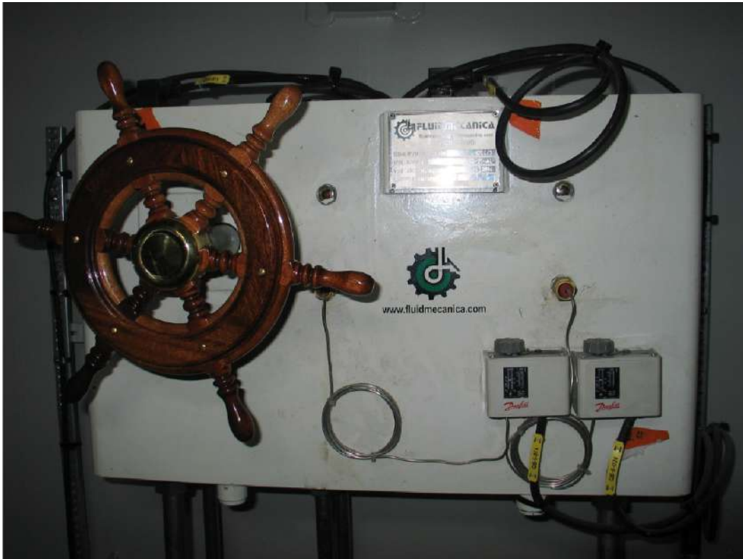
Figure 2-41 Steering Room - Oil Tank, Double with Emergency Manual Pump
