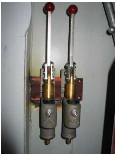
Figure 5-19 CO2 Room - FO Quick Closing Valves
