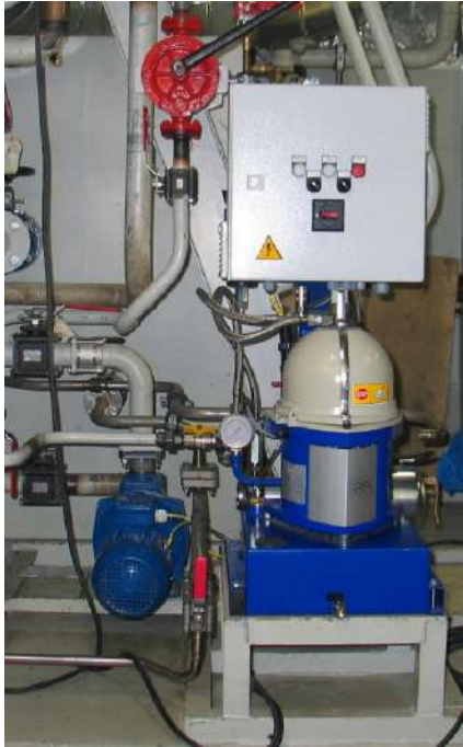
Figure 5-16 Port Engine Room - FO Transfer Pump and Centrifugal Separator
