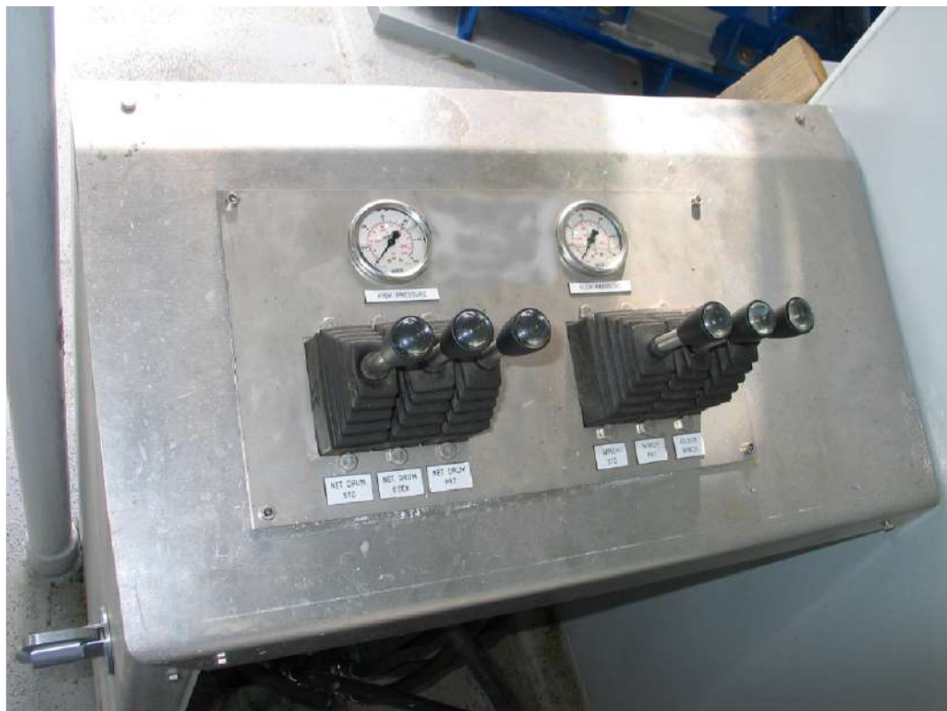
Figure5-48 Fishing Deck - Fishing Gear Deck Control Panel
