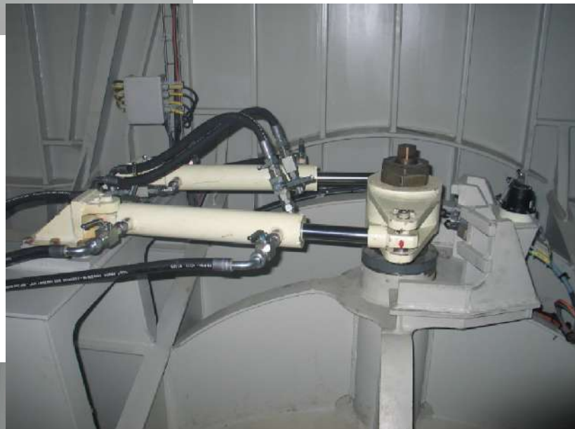
Figure 2-39 Steering Room – Rudder Stock & Steering Cylinders
