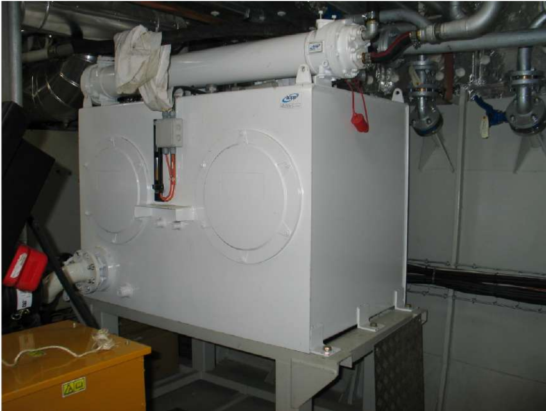
Figure 2-52 Engine Room - Oil Tank for Hydraulic Fishing Gear
