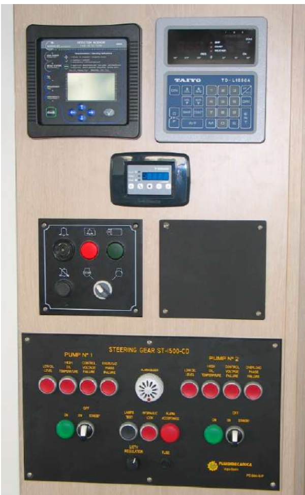
Figure 2-22 Wheelhouse - Aft Console
