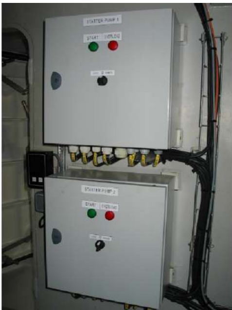
Fig5-1 Steering Gear - Electrical Starters HPU1 & 2
