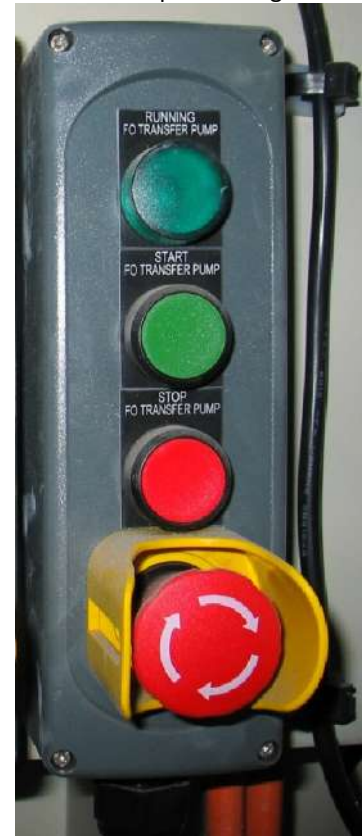
Figure 5-18 Engine Room - FO Transfer Pump Remote Control Panel
