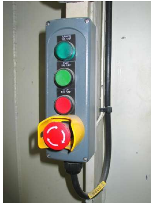
Figure 5-11 Workshop - Fire Pump Remote Control Panel
