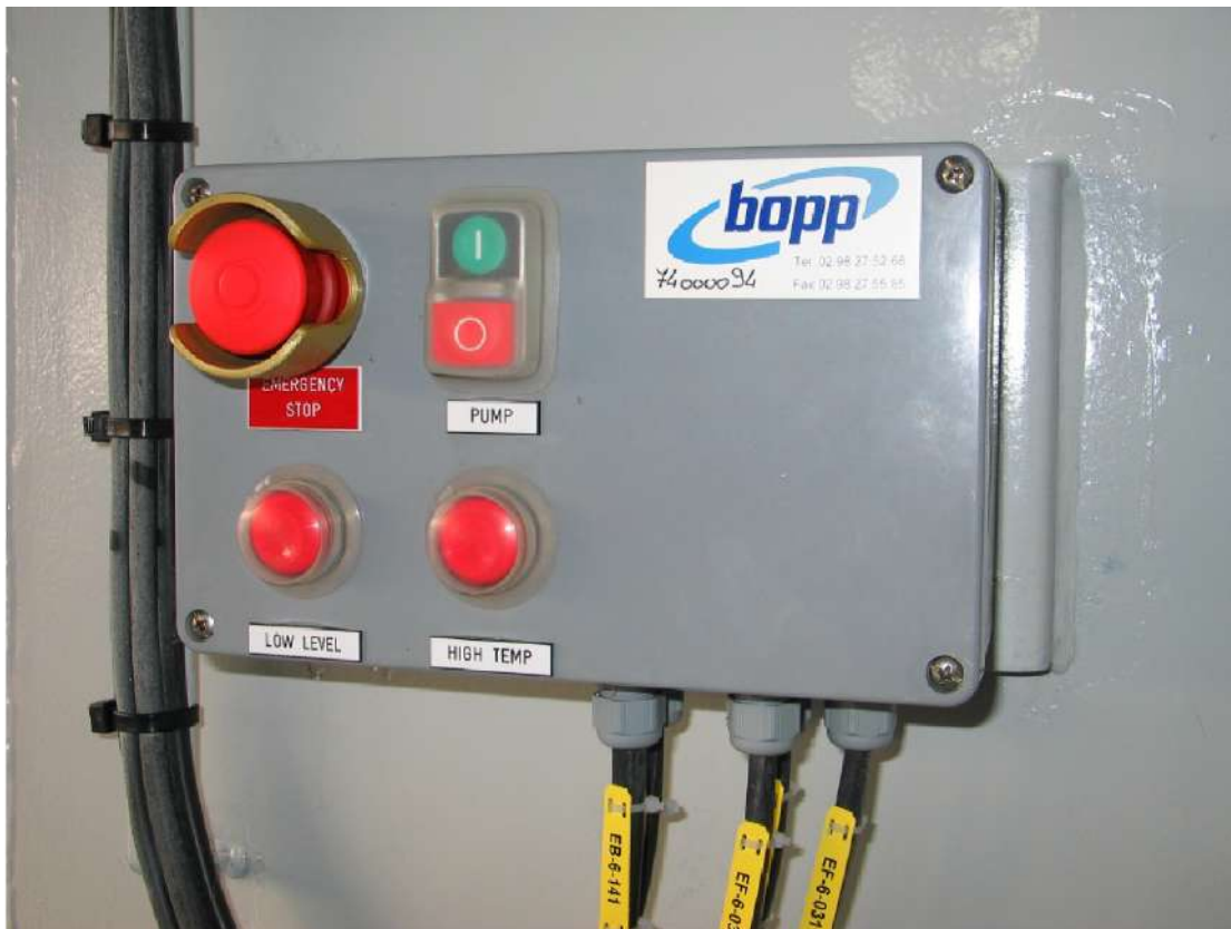
Figure5-47 Fishing Deck - Fishing Gear Electrical Panel
