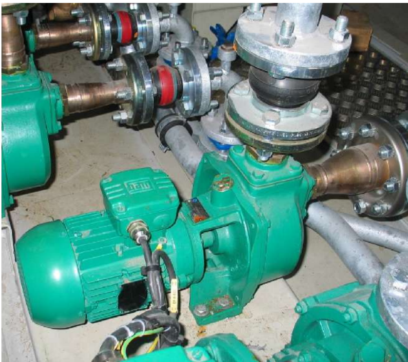
Figure5-44 Engine Room -Fishing Gear SW Cooling E-Pump
