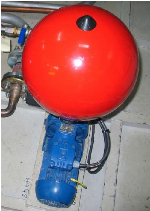
Figure 5-6 Engine Room - FW Pressure Pump
