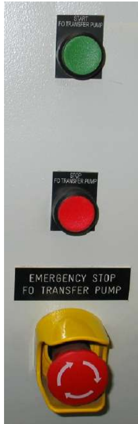
Figure 5-17 Main Switchboard - FO Transfer Pump Control Panel
