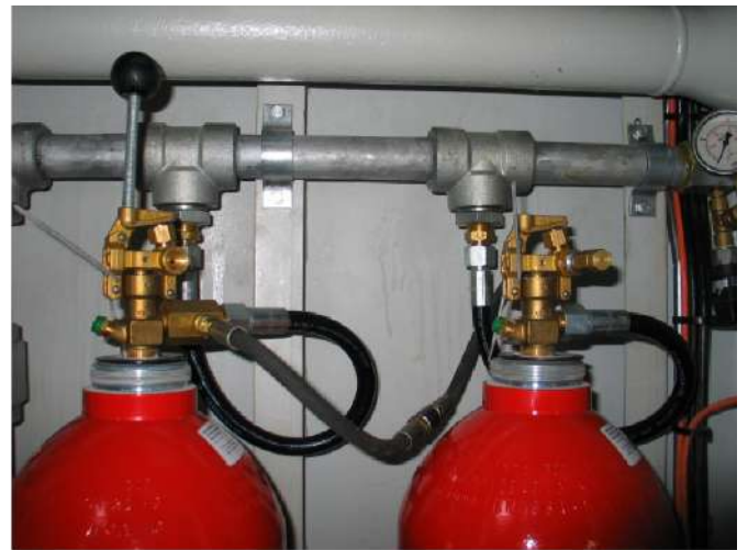
Figure 5-24 Mechanical Release Lever (Cylinder 1) and Pneumatic Release (Cylinder 2)
