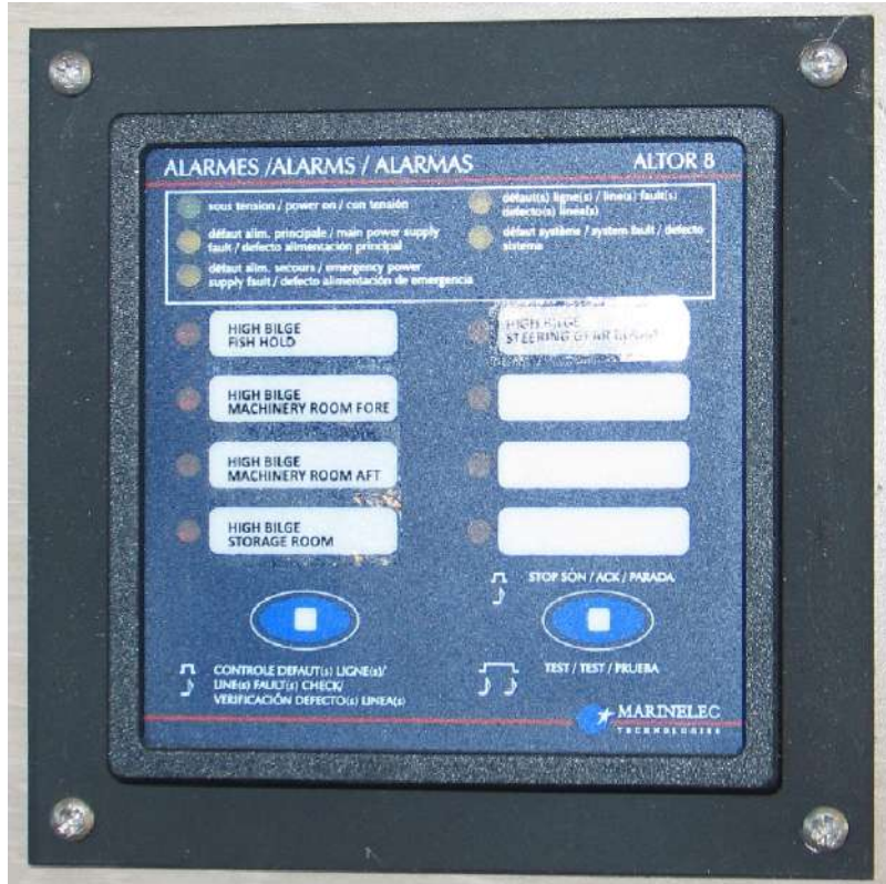
Figure 5-31 Bridge - Bilge Alarm Panel
