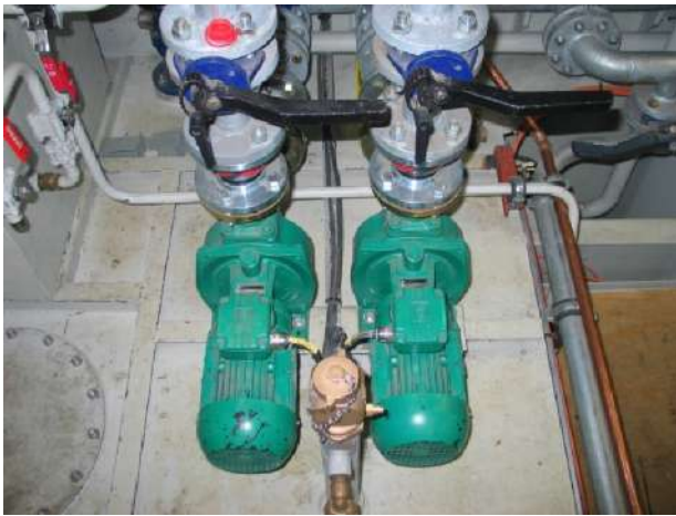
Figure 5-12 Engine Room - Bilge Pumps
