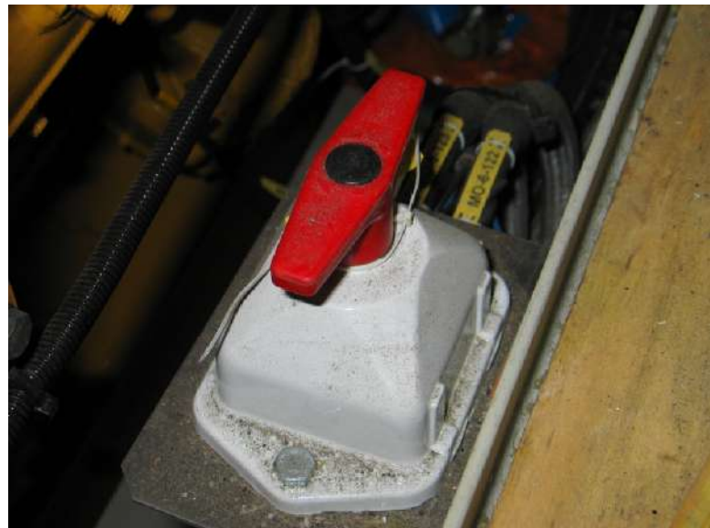
Figure 5-38 Engine Room - ME Battery Master Key
