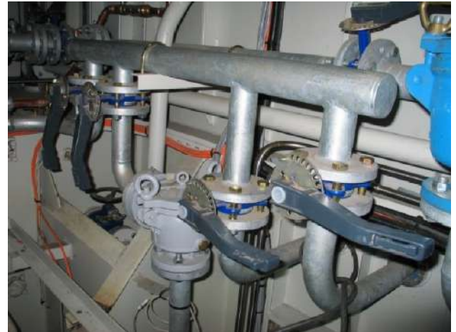
Figure 5-13 Engine Room - Bilge Manifold
