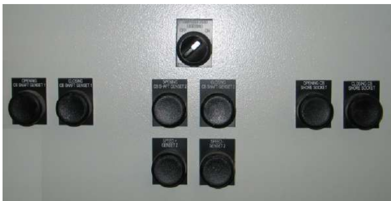
Figure 5-27 Main Electrical Switchboard - Production Cell
