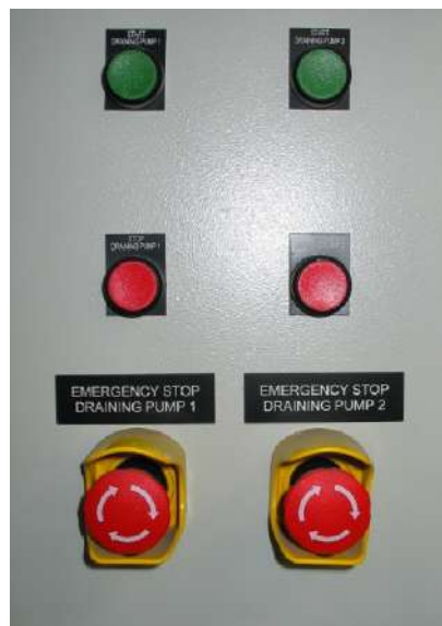
Figure 5-14 Main Switchboard - Bilge Pumps Control
