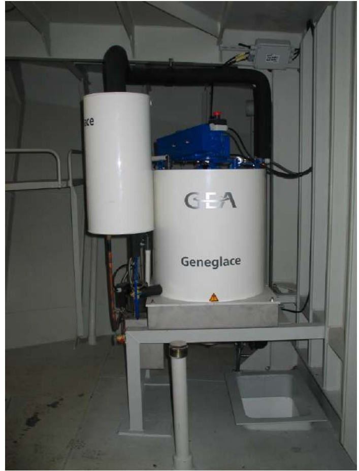
Figure 25 Fore Peak - Ice Generator
