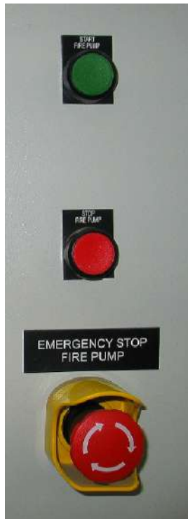
Figure 5-10 Main Switchboard - Fire Pump Control
