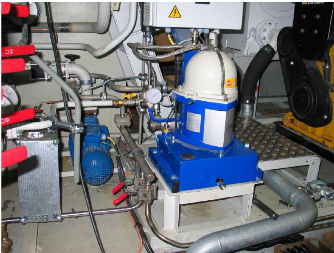
Figure 2-53 Engine Room - Fuel Oil Separator & Transfer Pump
