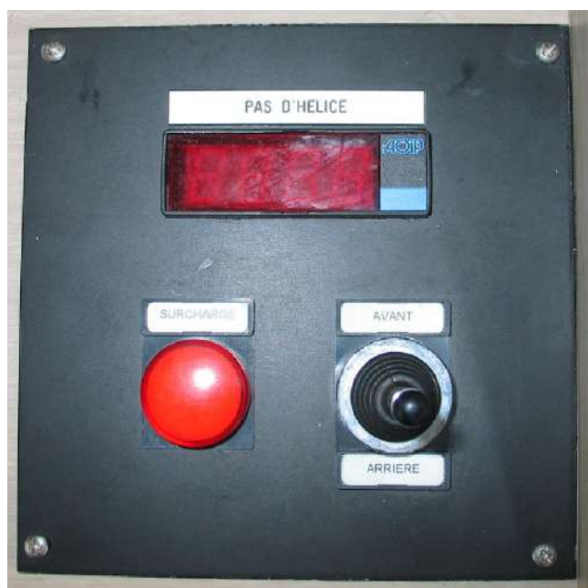
Figure 5-39 Bridge - Pitch Propeller Remote Control Panel
