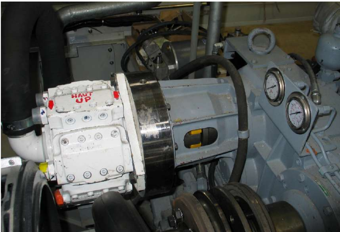
Figure 2-49 Engine Room - HP Hydraulic Pump for Fishing Gear
