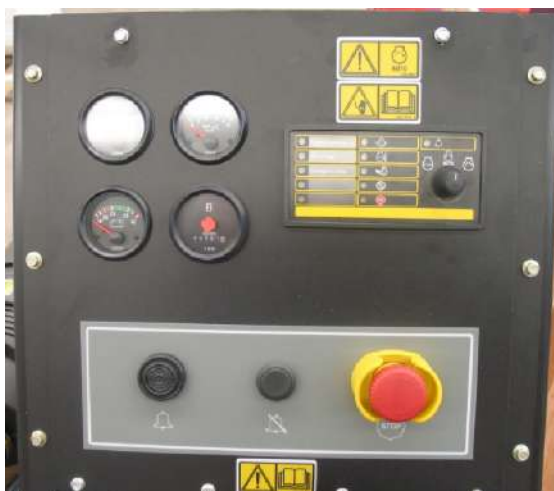
Figure 5-29 Genset - Control Panel
