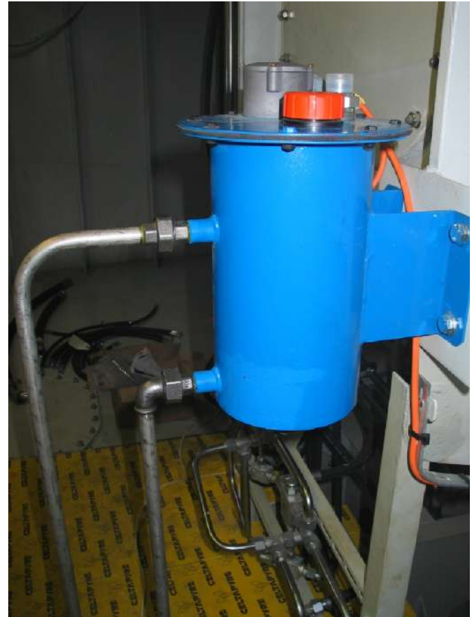
Figure 2-44 Storage Room - Fore Shaft Seal Lub Oil Tank
