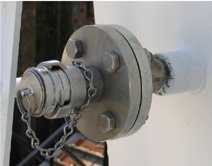
Figure 2-19 Stbd Upper Deck - Domestic Fresh Water Filling Connection
