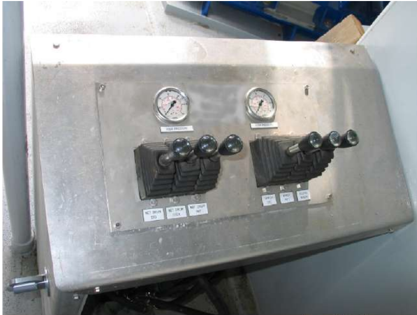
Figure 2-13 Fishing Deck - Fishing Deck Control Panel
