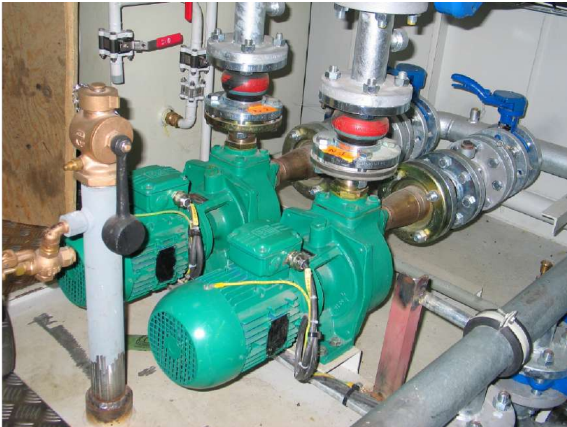
Figure 2-55 Engine Room - Sea Water Cooling Pumps for Fish Hold Refrigeration Unit
