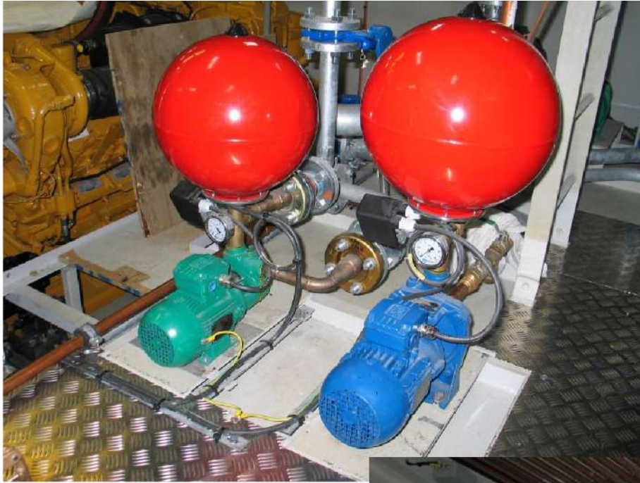
Figure 2-56 Engine Room - Sea & Fresh Water Pressure Pumps
