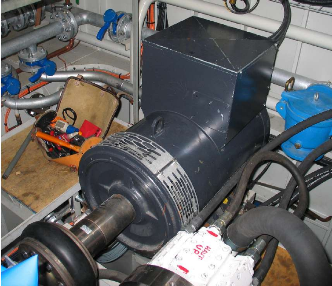
Figure 2-48 Engine Room - 100 kVA Shaft Generator
