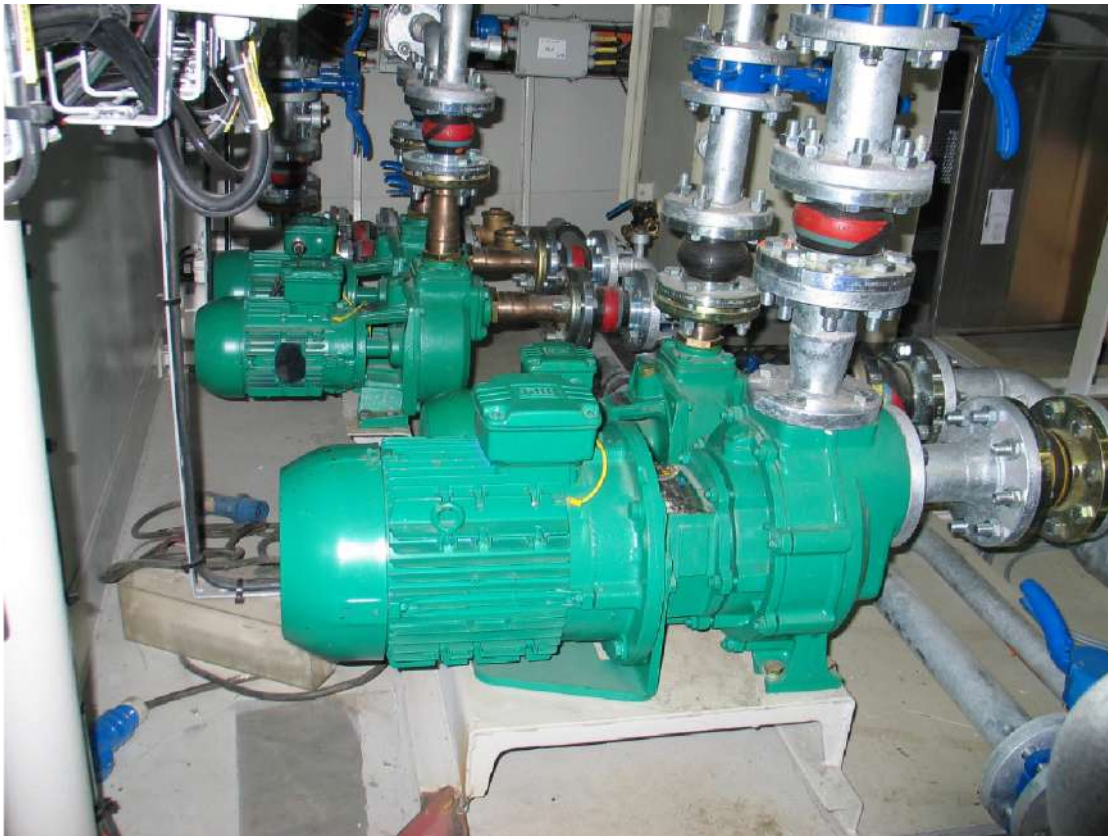
Figure 2-54 Engine Room - Fire Pump
