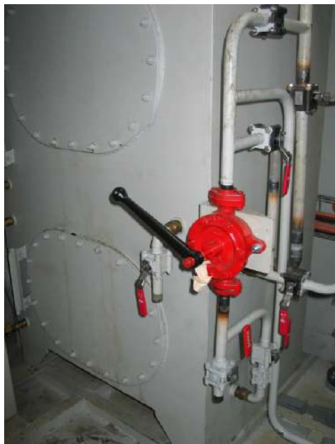
Figure 5-21 Stbd Engine Room - Lubricating oil Transfer Hand Pump
