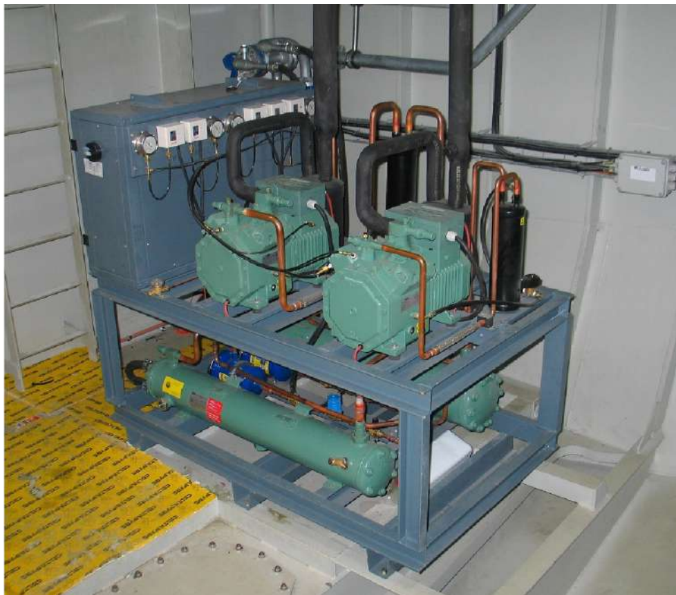
Figure 2-42 Storage Room - Refrigeration Plant for Fish Hold & Ice generator
