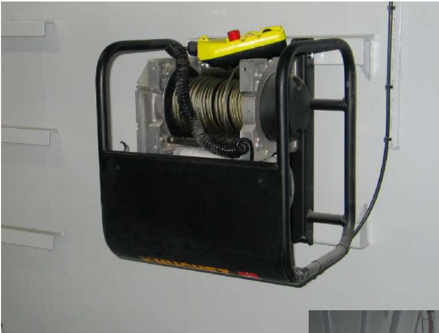
Figure 2-38 Fore Fishing Deck - Electric Winch for Hoisting Mast
