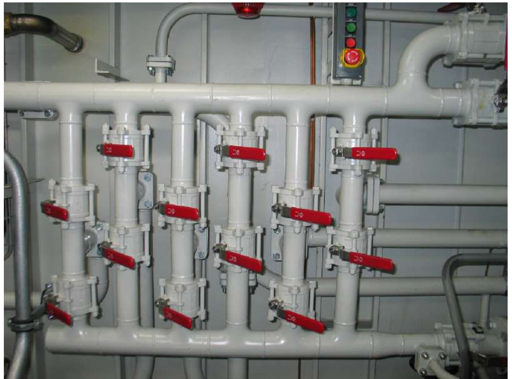
Figure 2-51 Engine Room - Fuel Oil Transfer Manifold
