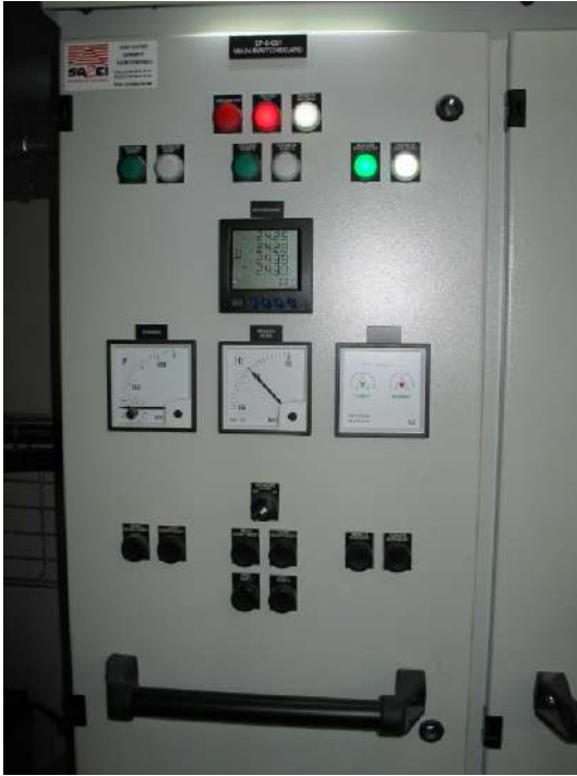
Figure 5-26 Main Electrical Switchboard - Production Cell
