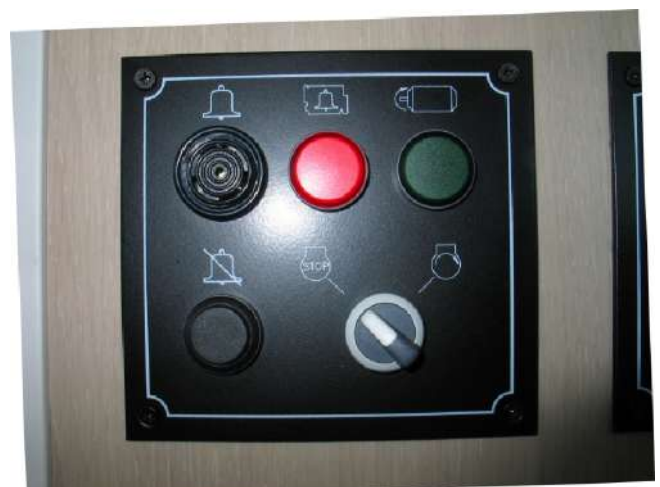
Figure 5-30 Genset - Bridge Remote Control Panel
