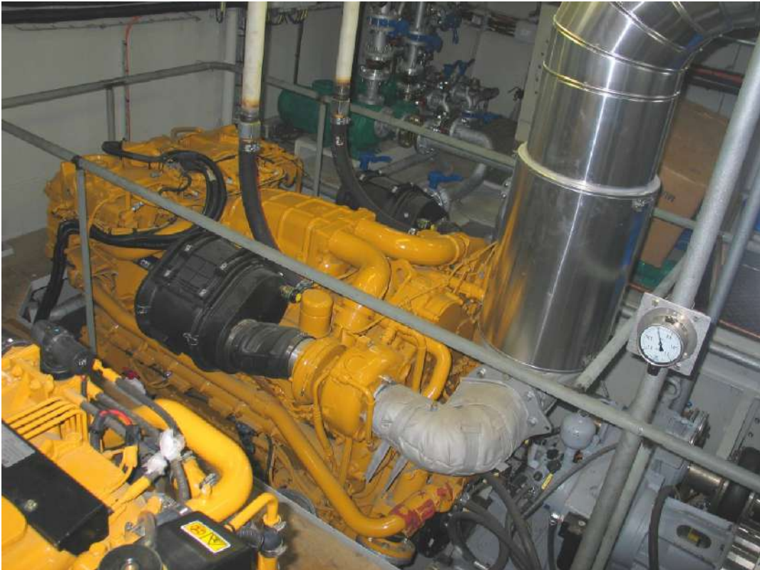
Figure 2-46 Engine Room - Main engine
