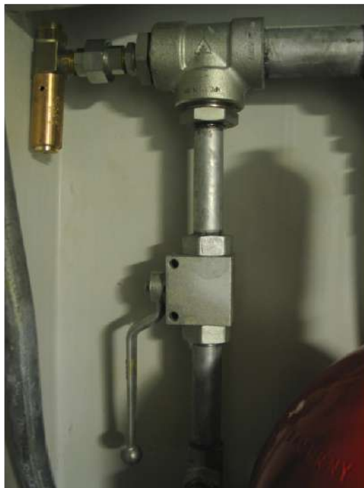
Figure 5-25 CO2 Isolating Valve
