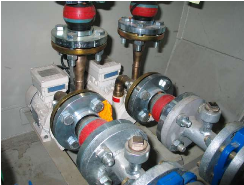
Figure 5-5 Stbd Engine Room - SW AC Cooling Pumps
