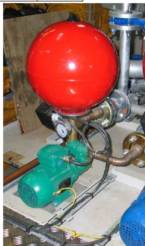
Figure 5-9 Engine Room - Sea Water Pressure Pump
