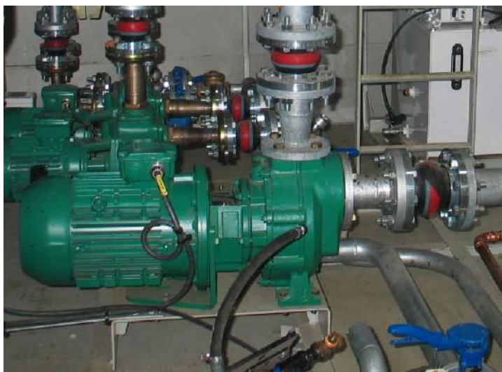
Figure 5-8 Engine Room - Fire Pump
